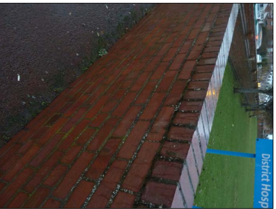
EXISTING SITE PHOTOGRAPH Existing masonry walls around site boundary. All walls around the site are to be demolished as part of the works. As many bricks as possible are proposed to be saved for re use as a full material for the new masonry brick columns. Bricks are to be salvaged and cleaned up for re use to build a new masonry brick column as shown to the south side of the new Care Hub site entrance off Mackenzie Avenue (refer to the plan below for the proposed location)
